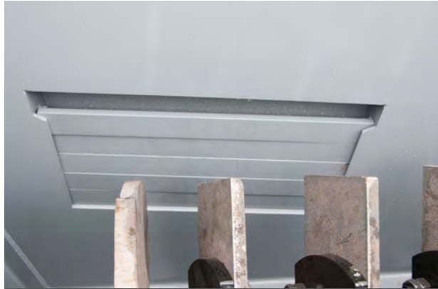
ADJUSTABLE OVERFLOW GATE
